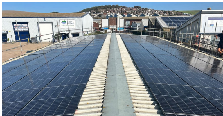
▲ The new solar array on the roof of the Newhaven Fish and Flake Ice Society is forecast to save the local industry over £230,000 over the next 20 years at current prices.
